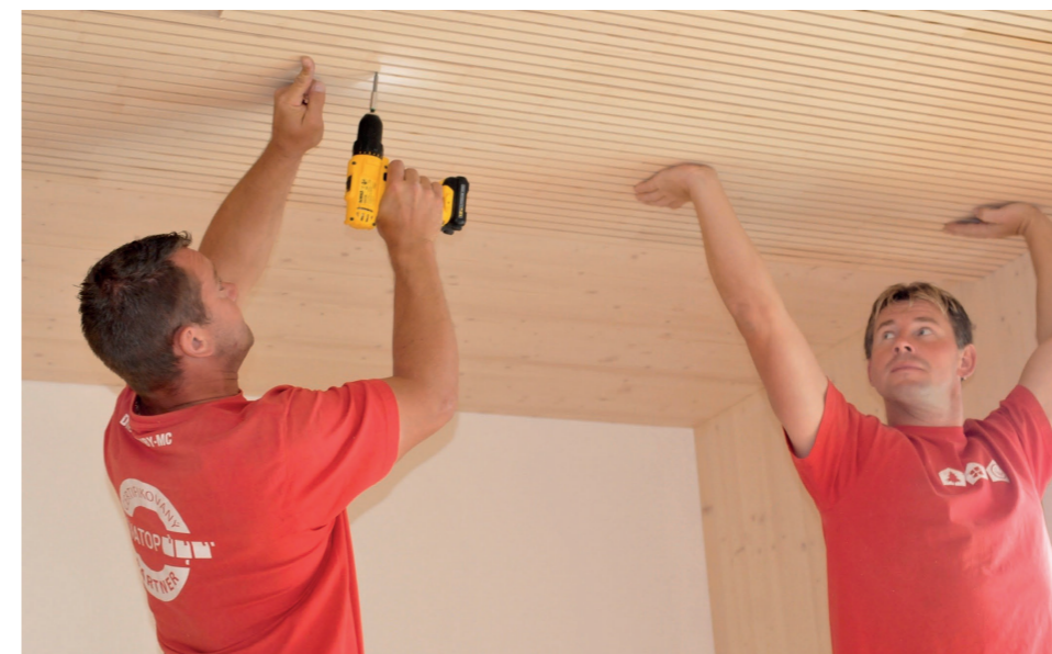
INSTALLATION OF THE NOVATOP ACOUSTIC CEILING BY MC FRAMES TEAM (COOPERATION OF EUROPEAN AND SOUTH AFRICAN BUILDES)
